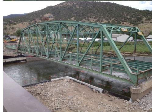
Example of causeways used on both sides of the river at the Dotsero bridge.
